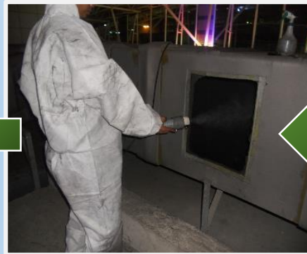
AIR DUCT SANITIZATION & TREATMENT
